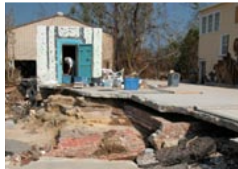
Damaged Historical Society building
